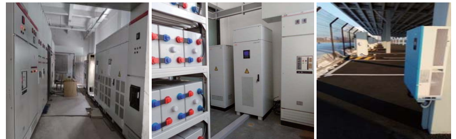
► BESS for EV Charger Station in Harbin
